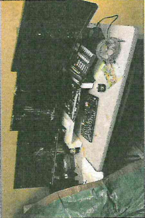
THE DAY AFTER New Year's a ceiling pipe burst inside Alpha Way's KVH Family Medicine-Cle Elum. The facility was back in operation by Monday, Jan. 7, with limited space due to ongoing repair work.
